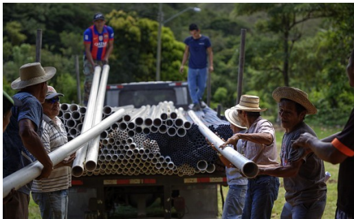
Community members in Las Delicias remove a shipment of PVC pipes from the delivery truck.
