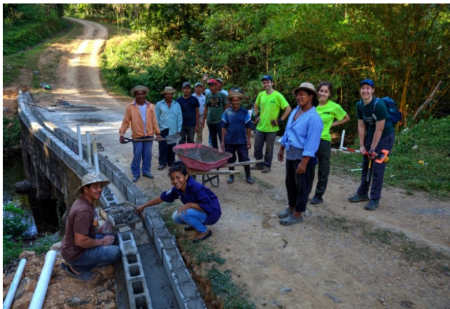
Photo from the Original Construction of the Above Ground Bridge Crossing from the March 2018 Implementation Trip.
