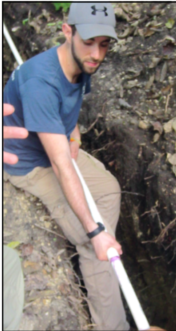
Alumni Ryan Gordon and Community Member Connecting Transmission Main | Photo: J. Schein
