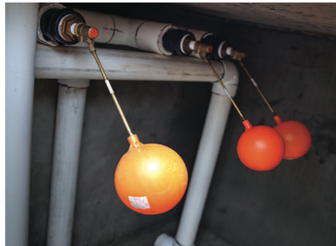
The float valves in a break tank. (December 2018)
